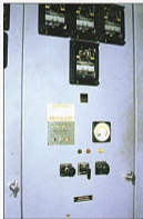
The insulation resistance tester display mounts in the switchgear panel. Readings are shown on a color-coded meter.
