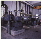
Each of three 250-hp, 480-volt centrifugal blower motors is monitored by insulation resistance testers.
