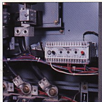
This Meg-Alert insulation resistance tester checks one of three 250-hp centrifugal blower motors. Each motor has its own tester.
